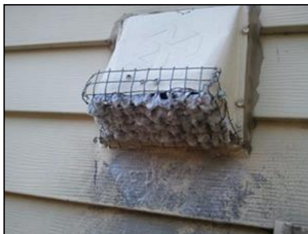
2. Dryer vent requires immediate and regular...
